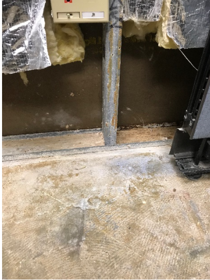
Figure 1: Room 122 Location of Stachybotrys Removed
