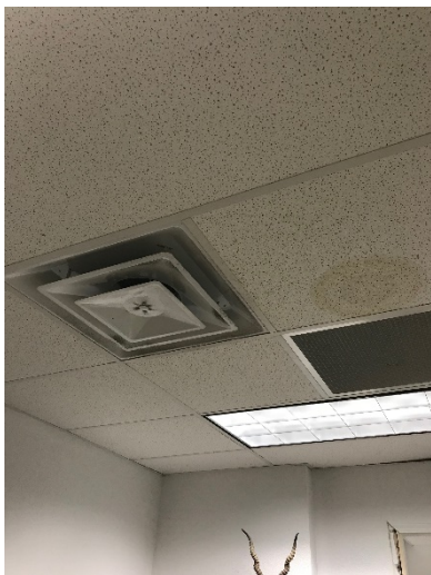
Figure 3: Room 127 Example of HVAC Register with Mold Present
